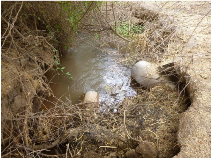
de Bont, Chris. Farmers has additional pipes to allow more water to flow into their canal. Mawala Irrigation Scheme, Tanzania . 2018.
